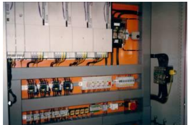
Figure 9: New constructed electrical cabinet, all Siemens material.
