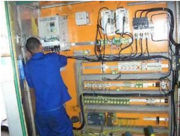
Figure 21: There are still a lot of wiring, but the main components are there. A small mishap. At 13.8. went by air freight of 30 KW motor with the controller to Angola. And various cables. Supposedly a week to 10 days. Today is 1.9. and there is not anything here! Fortunately, we have just delivered at the beginning with the first delivery, the replacement goods, in an emergency, we can then start. In Angola months for material you have to think in advance.
