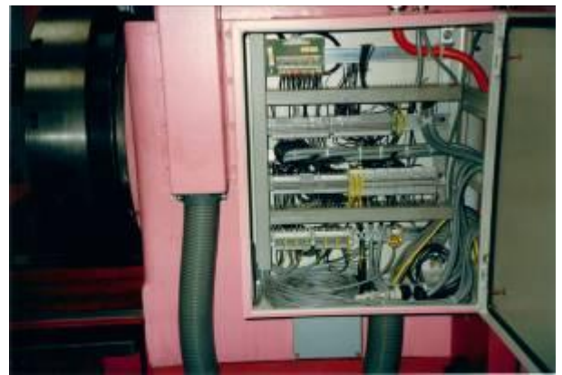
Figure 10: transmission electrical cabinet
