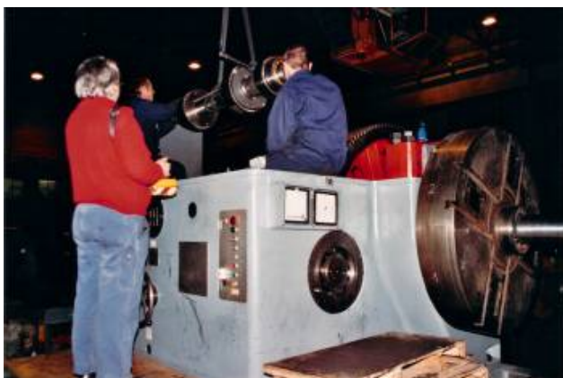
Finally the main gear shaft could be lifted out. Then we were able to offer the defective gear.
