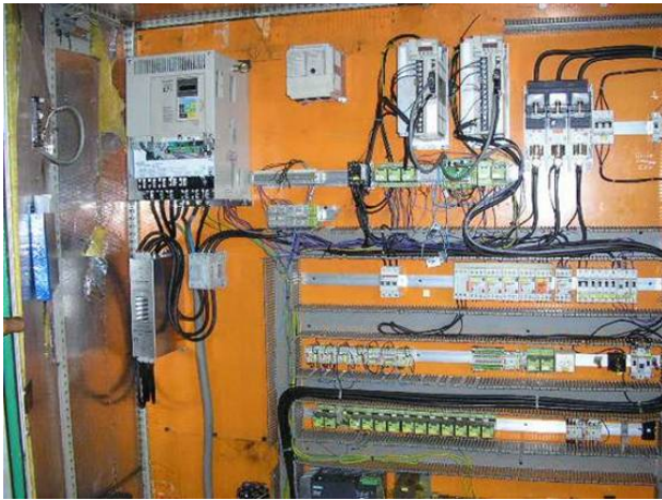
Photo 8: All that was cable away. (We had an idea, Wireles). The sources were too large, the machine had so much in it such as fairs, break monitoring Driven tools C axis. But you never brauchet it. The machine was fully occupied with pipe turning, so we have only the bare minimum before it for maintenance.
