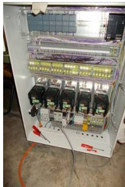
For all motors of the units we have built, each with 0.75 kW instead of protecting equal to 5 pieces of frequency. These can be adjusted continuously. From 0 to 70 Hertz, the option of up to 100 Hz. I.e. twice the speed. Above the S7- 1200 is arranged. WU5140c
