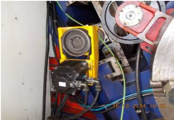
The whole was treated with a Z drive sub-reduction 1: 2 Construction WIAP renewed.
