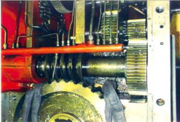
The whole longitudinal slide feed drive, which drive the rack was completely phased out. WU4310
