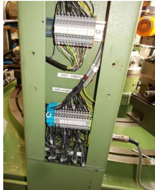
On the side of the column to the terminals for the external panel. So that when a cable break to have to solder without the cable can be replaced quickly. WU5140
