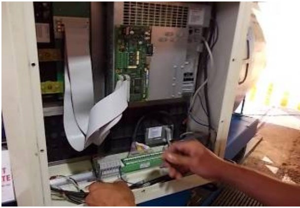
Significantly less cables that hang around there. Sure, only about 30%.WU_232_290
